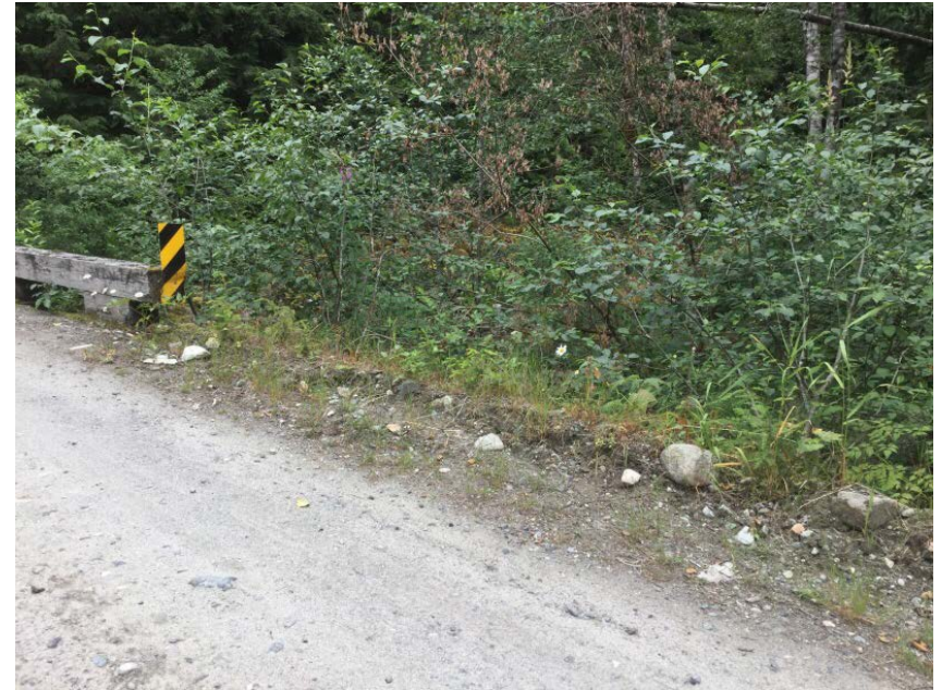
Missing upstream left approach fender - rolled off road
