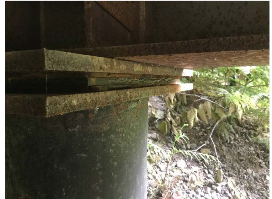
Left bank, downstream bearing pad weathering
