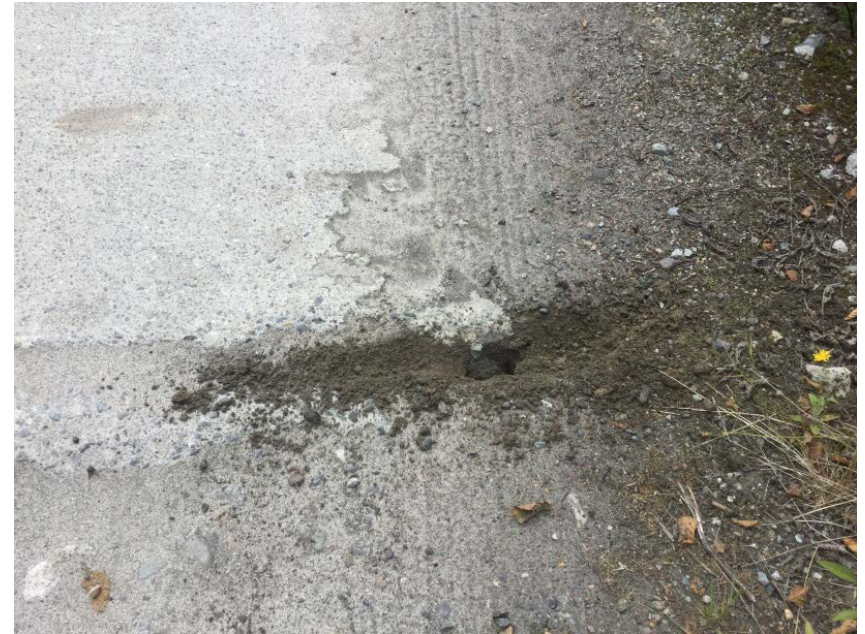
Deck damage at right approach
