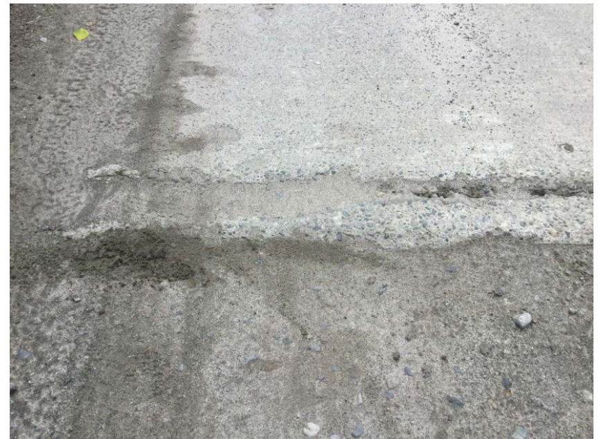
Ballast wall damage at right approach
